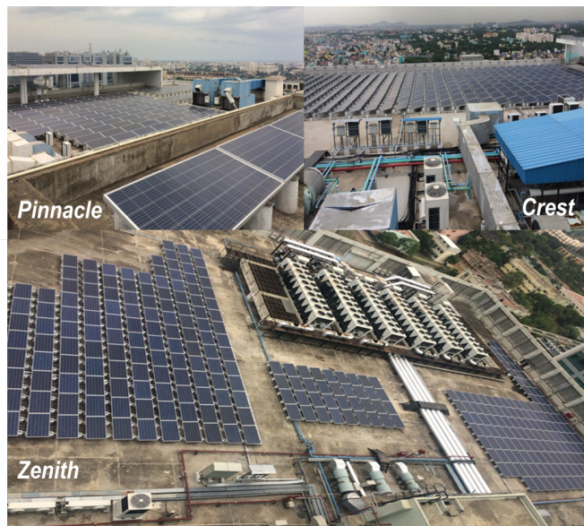
Figure3. Rooftop Solar PV installed at Pinnacle, Crest and Zenith building at Ascendas
