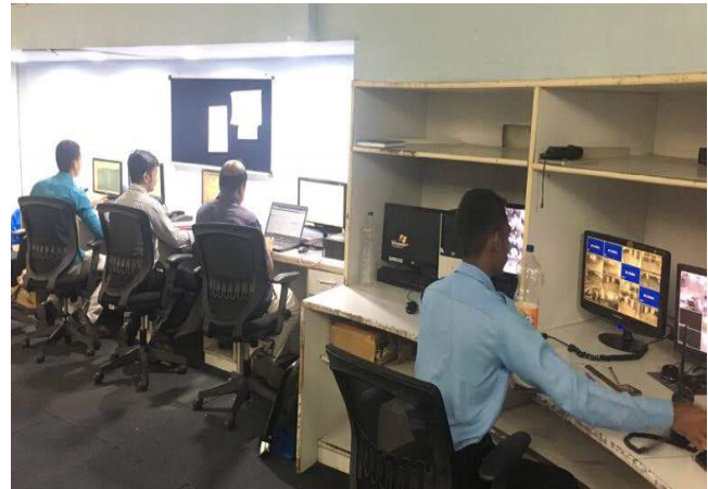
Figure1. Building Management System Control Centre
