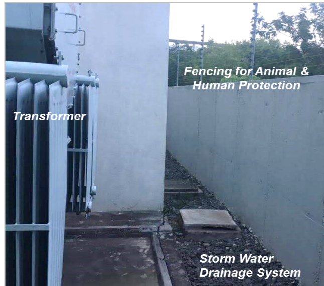
Figure2. Protected substation transformer at Ascendas
