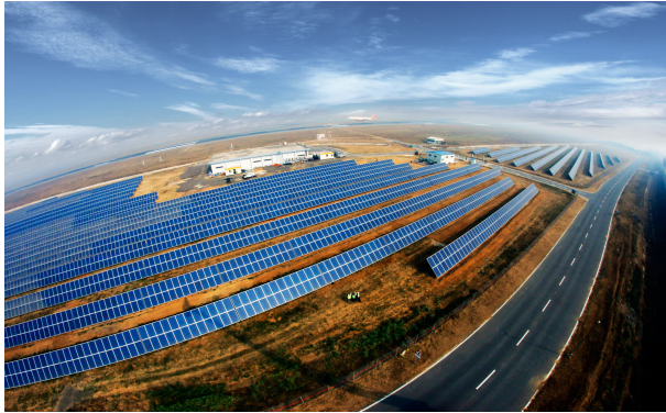
Figure 2. 7.8MW Solar Power Plant at IGIA
