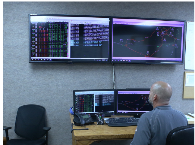
Figure 1. Glasgow EPB SCADA system
