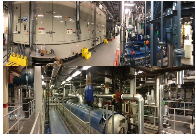
Figure 1. Gas turbine, Heat recovery steam generator and boilers inside the Main campus Energy building
