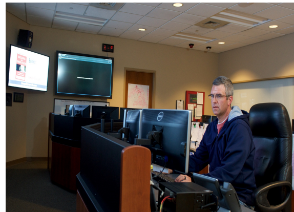
Figure 1. Nolin RECC - OMS integrated SCADA systems
